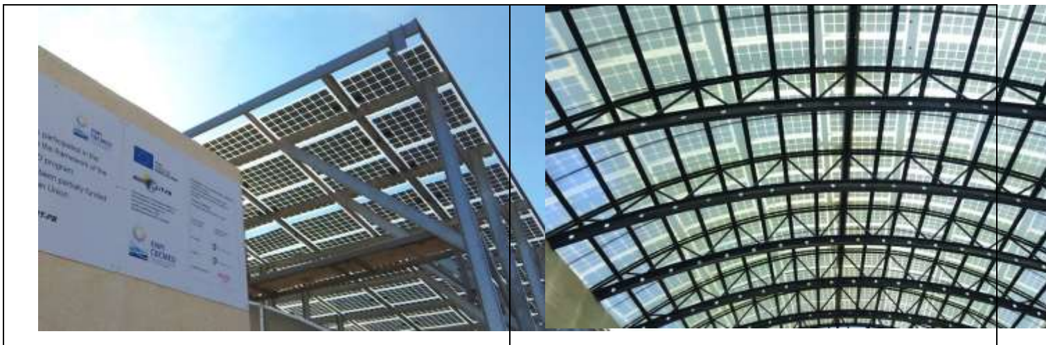
Photovoltaic Solution Package at BAU
